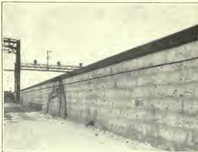
FIG. 277. TRACK ELEVATION. Masonry retaining wall of the Chicago & North Western Railway at Kinzie Street and North Francisco Avenue.
